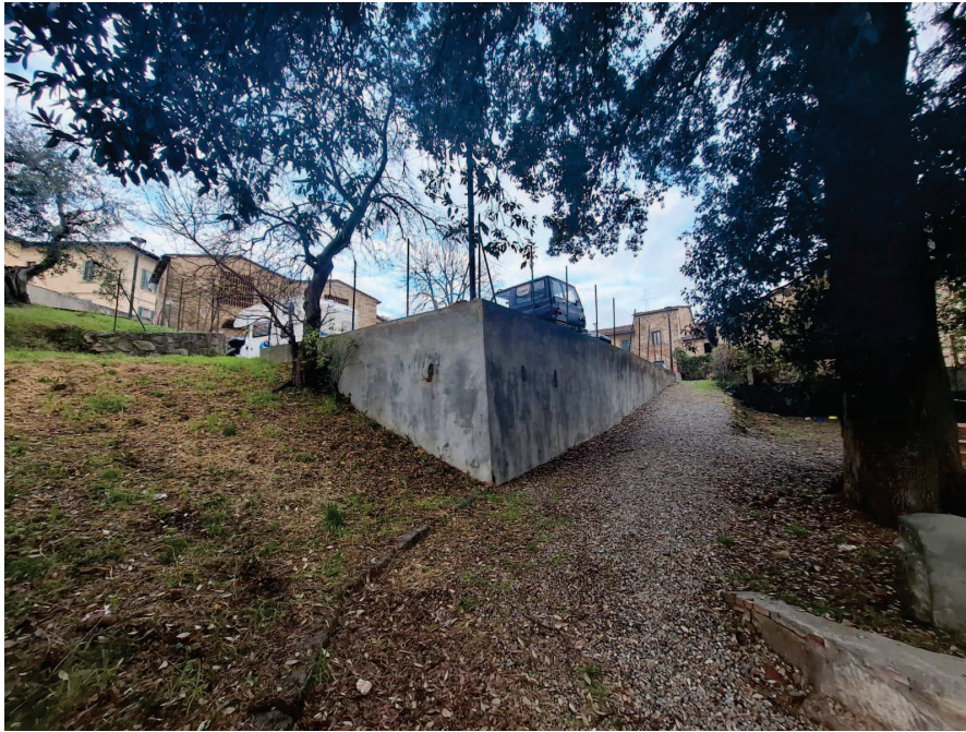
Fig 18 - Lack of stairs
